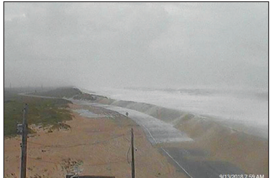
The washout at the S curve at Mirlo Beach, Rodanthe, after Hurricane Florence (Reprint from NC DOT NC 12 Facebook)
